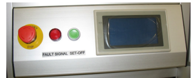
The Touch Screen Operated Control Panel
